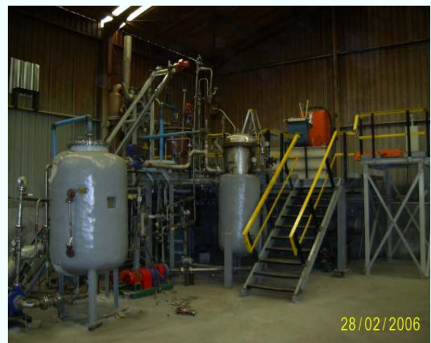
Gold potassium cyanide manufacturing facility
