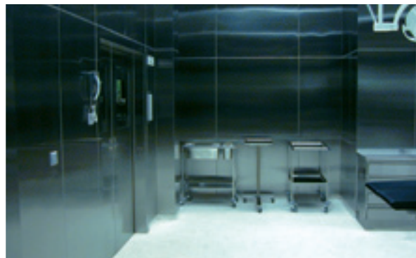
operating theatre made entirely of stainless steel 0H18N9
