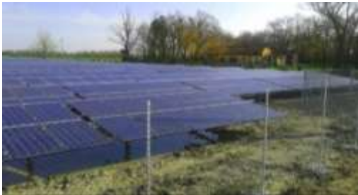
Copparo, 1 MWp Italy
