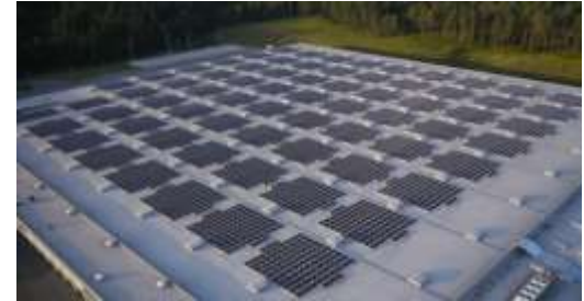
Hofer Logistics Centre, 2 MWp Slovenia
