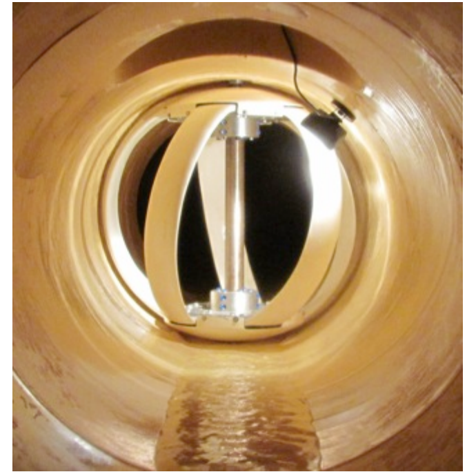
LucidPipe Installed Lemona Booster Station - Riverside, CA
