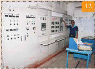
Kiln Control Room
