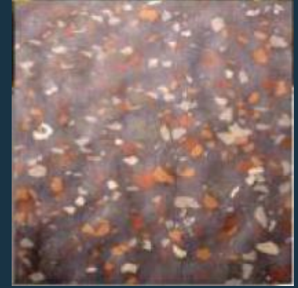
HAMMER BLOW SURFACE
