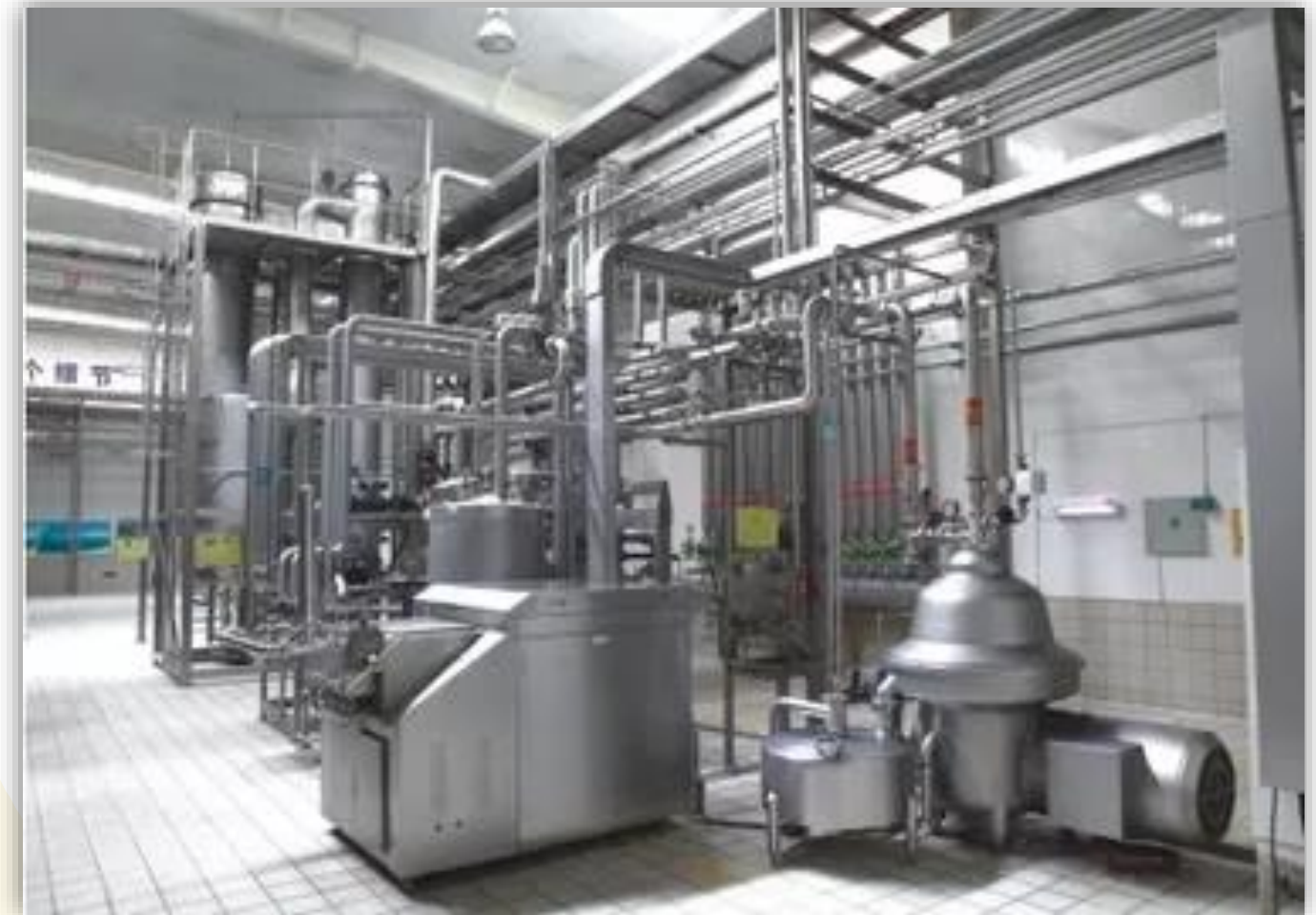
New UHT line-3 installment in Q1, 2023, beverage capacity up to 120M liters (i/o 60M previously)
