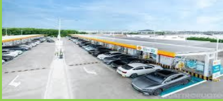
Recharging Platform for 2 to 12 Vehicles Recharging
